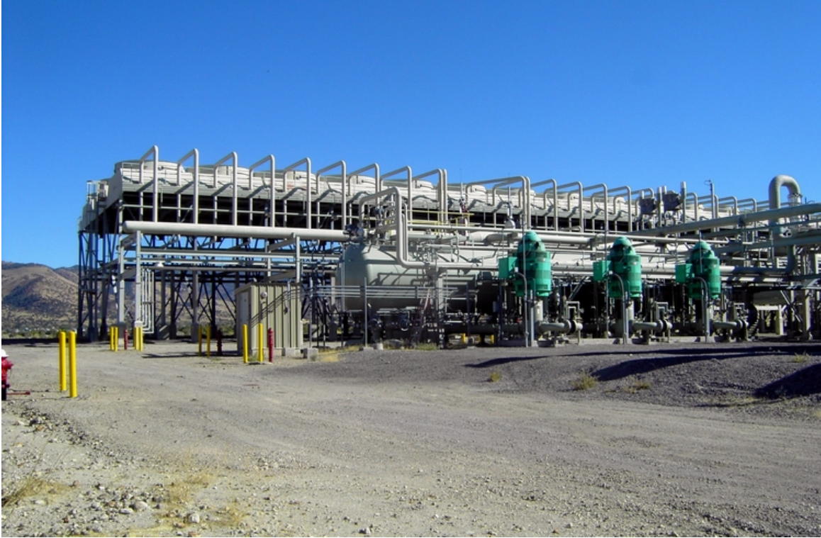
Figure 3. A section of the ACCs at the Steamboat 2 binary power plant in Nevada. Photo by R. DiPippo.
